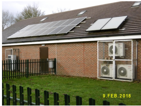
Air Source heat pumps and Solar Panels
