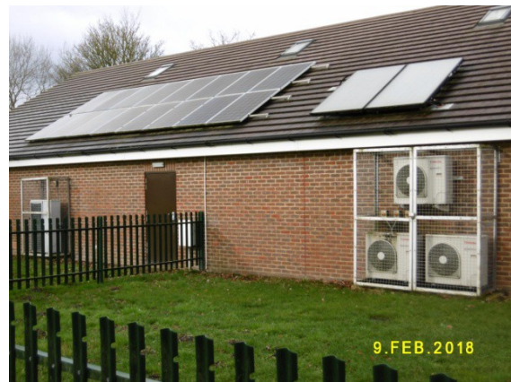
Air Source heat pumps and Solar Panels
