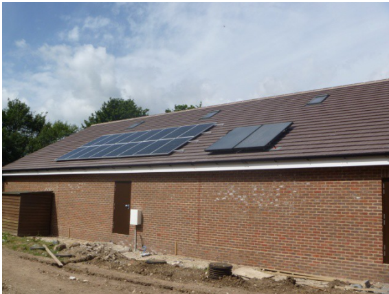
Above Solar thermal and PV panels
