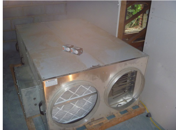
Heat Recycling Ventilation plant
